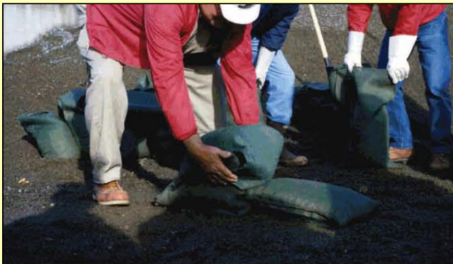
Fill bags ½ full. Fold open end of bag under & lay pointing upstream, butting bags end-to-end.
