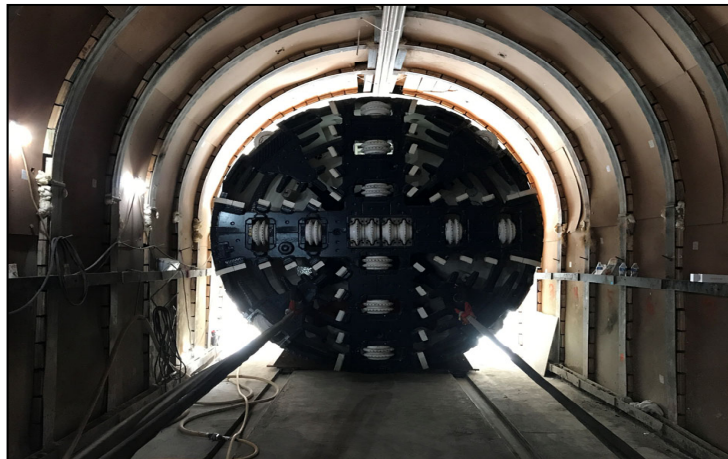
River Supply Conduit Upper Reach Improvement Unit 7 (RSC7) will install 13,325 feet of 78-inch welded steel pipeline, and the entire RSC Upper Reach will connect the North Hollywood Pump Station to Headworks.
