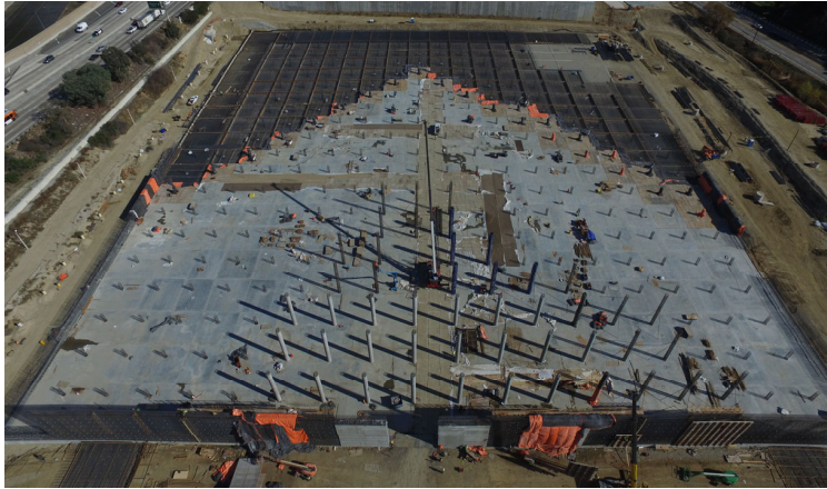
Headworks Reservoir West is under construction and is 95% complete. The massive network of steel rebar and the “chevron” concrete pour pattern was implemented to reduce cracking.
