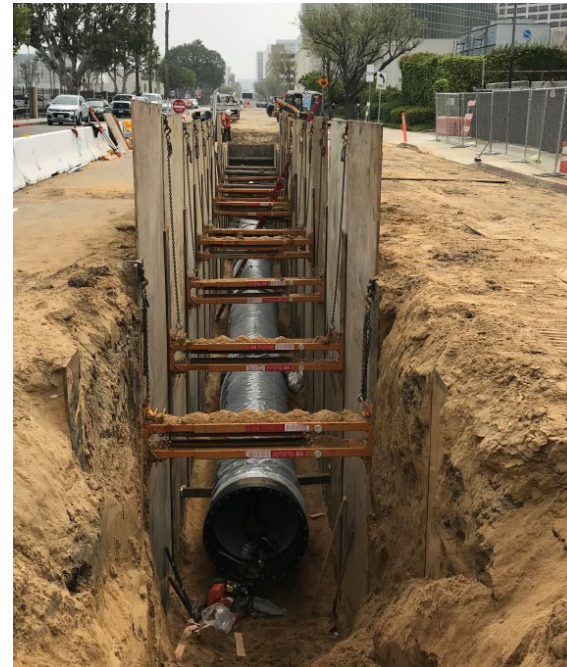
The Century Trunk Line Unit 1 Project will install approximately 10,800 feet of new 24-inch and 48-inch earthquake resistant ductile iron pipe. Phase 1 groundbreaking began in February 2020 and a total of 5,930 square feet of trunk line has been completed.
