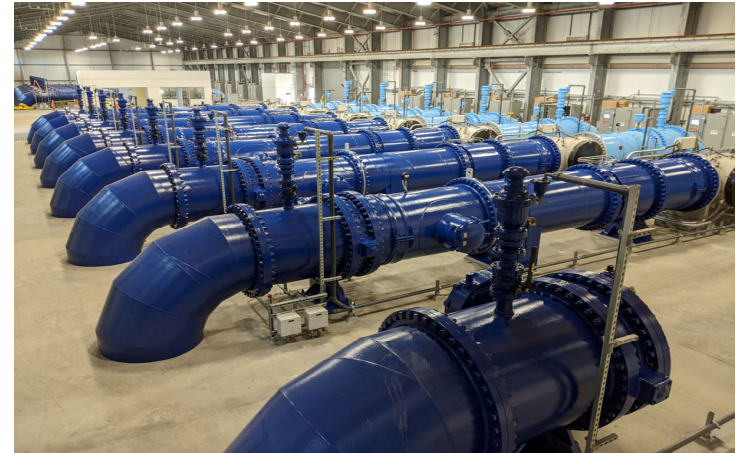
The LA Reservoir UV Treatment Facility is a 650 million-gallon-per-day treatment plant to meet water quality regulations and is 92% complete.
